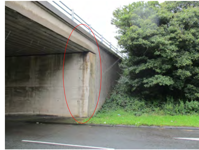
Photograph 5 North Abutment- Staining at bearings
