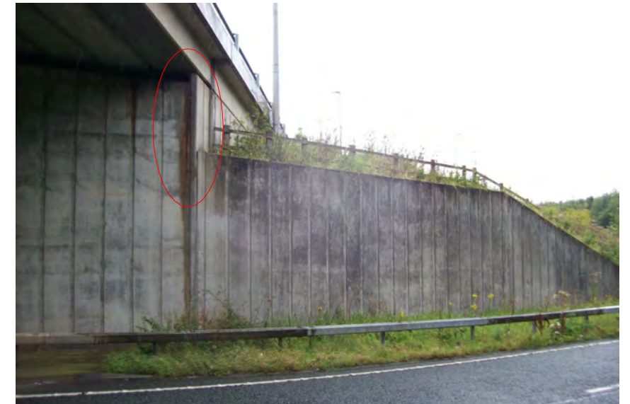
Photograph 2 South elevation- Staining due to water leakage at joints
