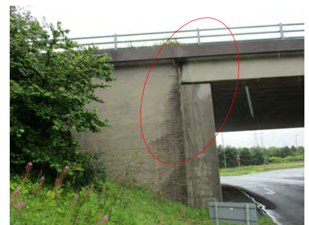
Photograph 3 North Elevation- Staining due to water leakage
