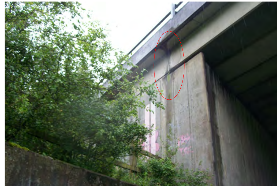
Photograph 4 South Abutment due to water leakage
