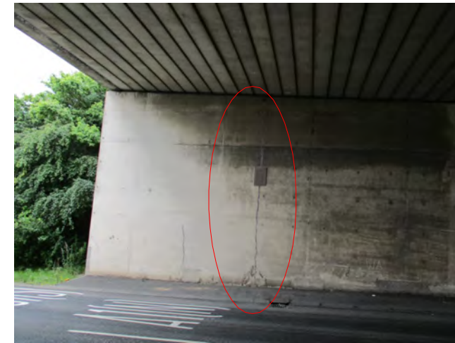
Photograph 6 Vertical crack on the abutment wall
