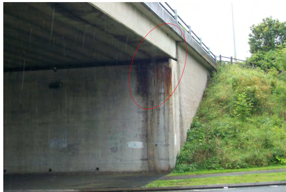
Photograph 5 North abutment- Staining due to water leakage
